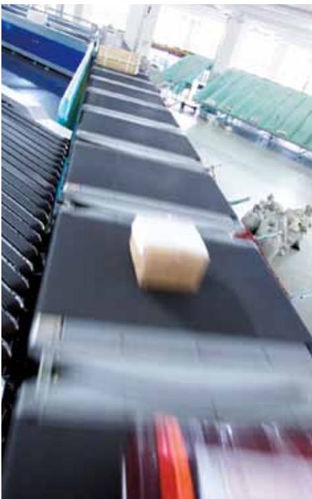
Lateral sorter in a distribution centre. The high acceleration requires the belt surface to have an extremely high coefficient of friction.
