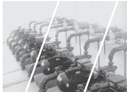
Boosting and Distribution of surface water
